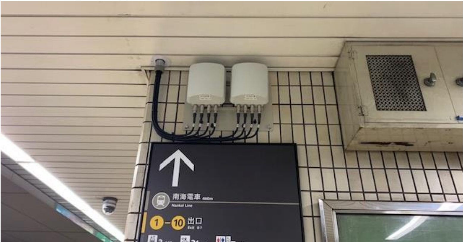
Passengers' communications inside tunnels
